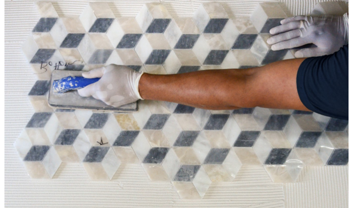
Step 4 To achieve the flattest possible surface, lightly tap the sheets using light pressure with a grout float or a wooden beating block and a finish hammer. To unify sheet transitions, tap from one sheet to the next.
