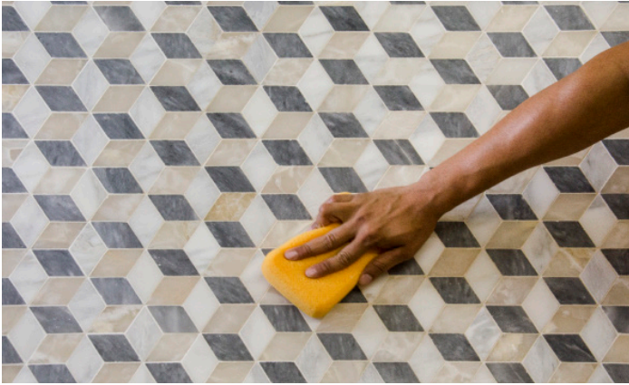
Step 9 Allow grout to set until firm and smooth finish with a damp sponge. After approximately 2 hours, remove grout haze with a lightly damp sponge.
