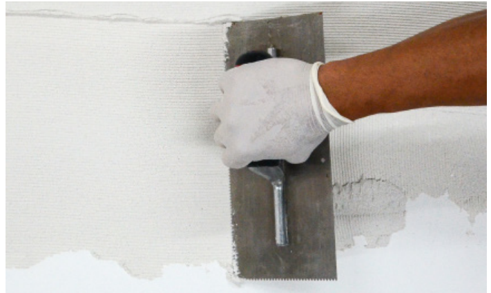
Step 2 To establish the proper depth of the setting bed, use a 3/16" x 1/4" v-notch trowel to apply additional thinset and comb full notches in one direction.
